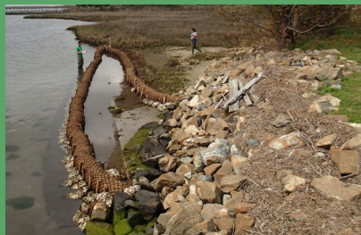
Installation spring of 2014
