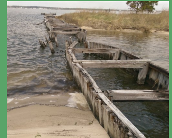
May 2018 breached abandoned sluice
